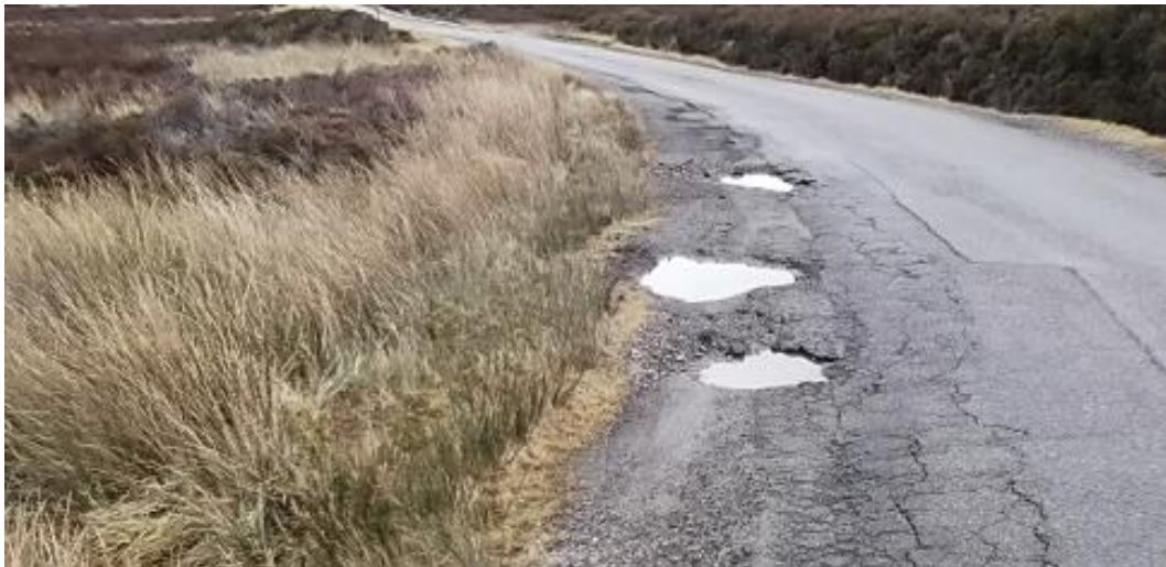
Typical Road Failure
