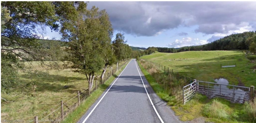
Typical edge damage, lack of passing places and poor drainage
